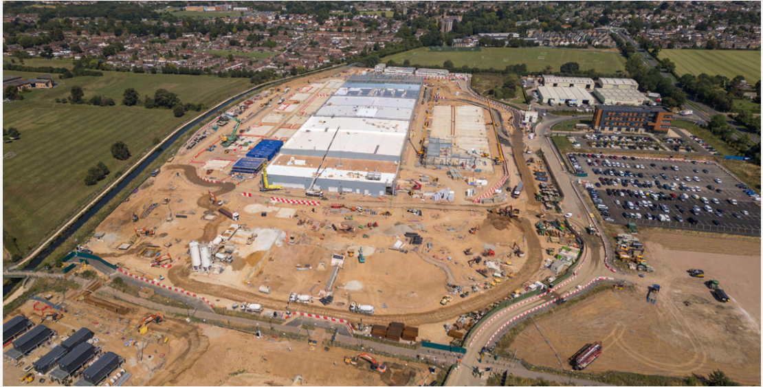
This $1 billion Google data centre, under construction north of London, gives a sense of the scale of the computing facilities now going up all over the world.
